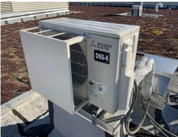
9 - DUCTLESS SPLIT SYSTEM
