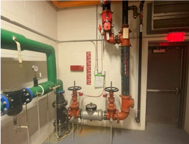
13 - SPRINKLER BACKFLOW PREVENTER
